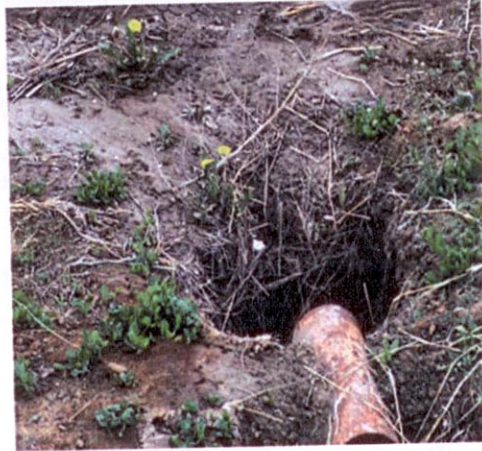
Figure 11: Erosion from simple pipe diversion
