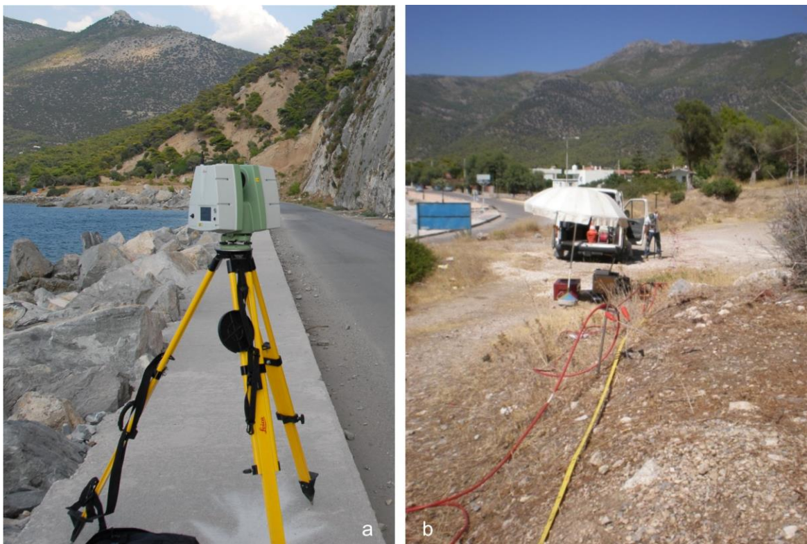
Figure 3. Field work data acquisition by surveying with the terrestrial laser scanner at the station SG-2 (a) and geophysical tomography along the ERT-1 section (b).
