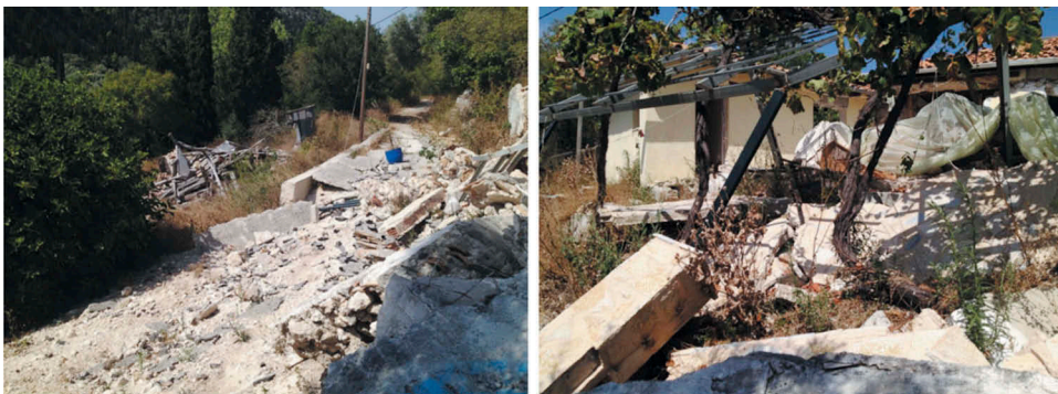
Figure 8. Field photographs (July 2016) showing structural damage imposed by an earthquake-induced landslide at Dragano.
