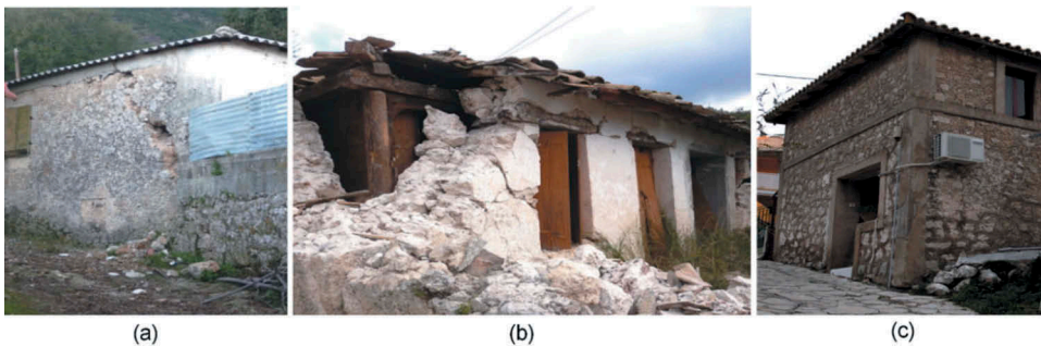
Figure 14. (a) LBSM “Yellow” tagged building in Agios Petros; (b) Damage of a single floor LBSM-TC in Athani; (c) LBSM-RC in Kalamitsi remained intact after the earthquake.
