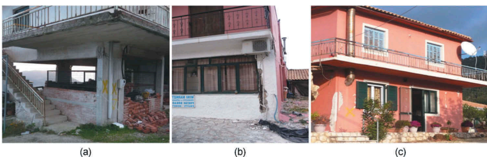
Figure 12. Damaged RC buildings in Athani: (a-b) Damage to columns and beam column joints at RC buildings; (c) Large cracks at infill panels.
